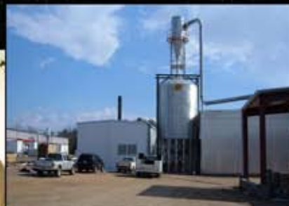
Silo with Unloader
